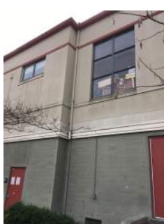
REPLACE ENTIRE DOWNSPOUT
